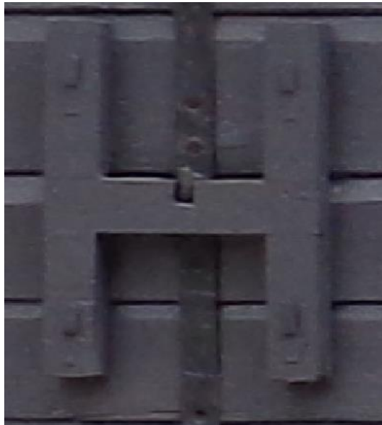
French side lower – an adjustment had to be made to accommodate for the metal framework.
